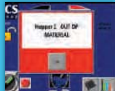
Audible and visual alarms are clearly identified on the display panel.
